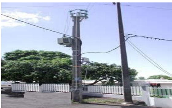
Pole mounted substation
